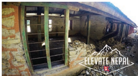
One of Elevate Nepal's upcoming projects is to fund the rebuilding of a 700-student primary school in the village of Sarsyu.
